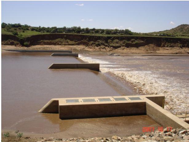
Figure 9: Multi Notch Crump Gauging Weir (photograph by Jackie van Bosch, DWA, South Africa)
